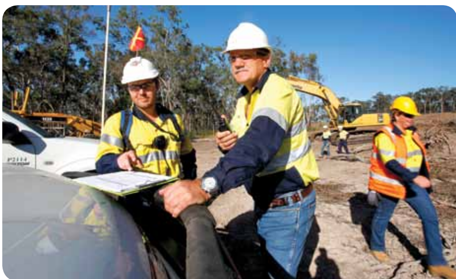
ACTION STATIONS: Clearing has been completed and civil works continue to prepare the site for the construction of the LNG facility.
