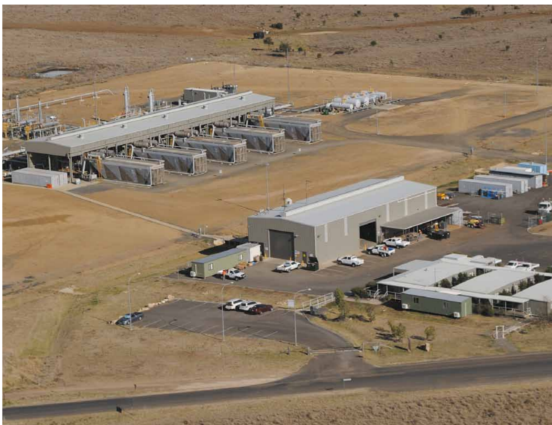
Australia Pacific LNG's operating gas processing facility at Spring Gully, near Roma
